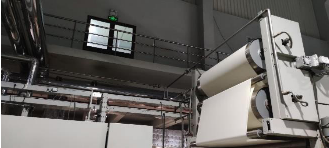
Figure 11. Cooling water pipeline for stenter machine
