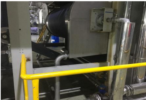
Figure 12. Cooling with water at a continuous machine
