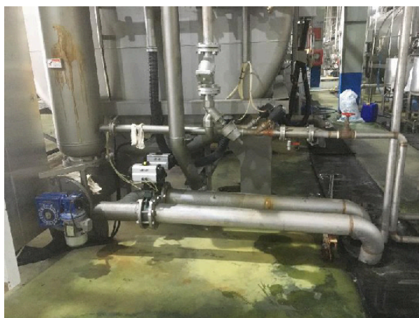
Figure 8. Heat exchanger and cooling water pipeline to the storage tank for circulation
