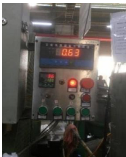
Figure 6. 4-level automatic water supply system at a factory
