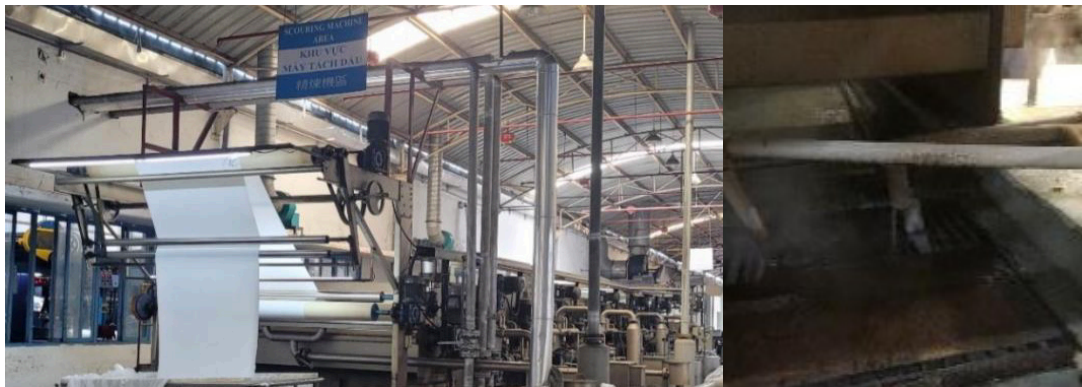
Figure 16. Recovering condensate from an oil remover
