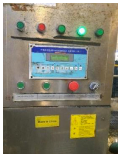
Figure 7. Automatic water supply controller at a factory
