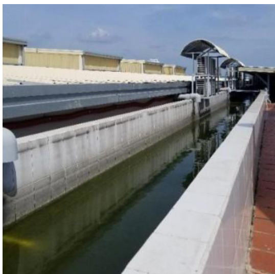
Figure 34. Typical factory rainwater filtration system
