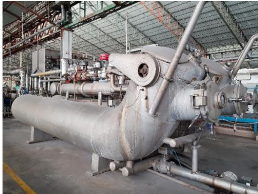
Figure 14. Recovering condensate from Jet machines
