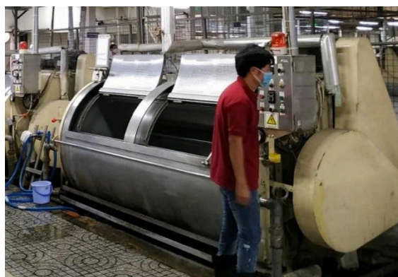
Figure 5. Manual water supply washing machine at a factory
