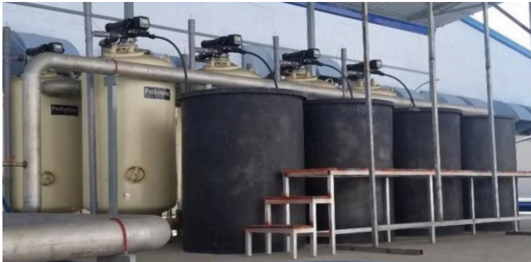
Figure 35. Typical factory rainwater filtration system
